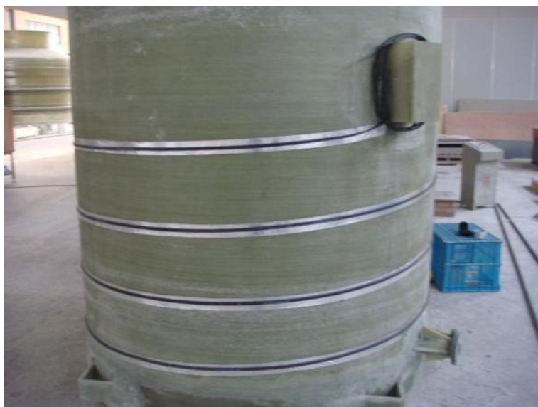
Tank With Heat Tracing System
