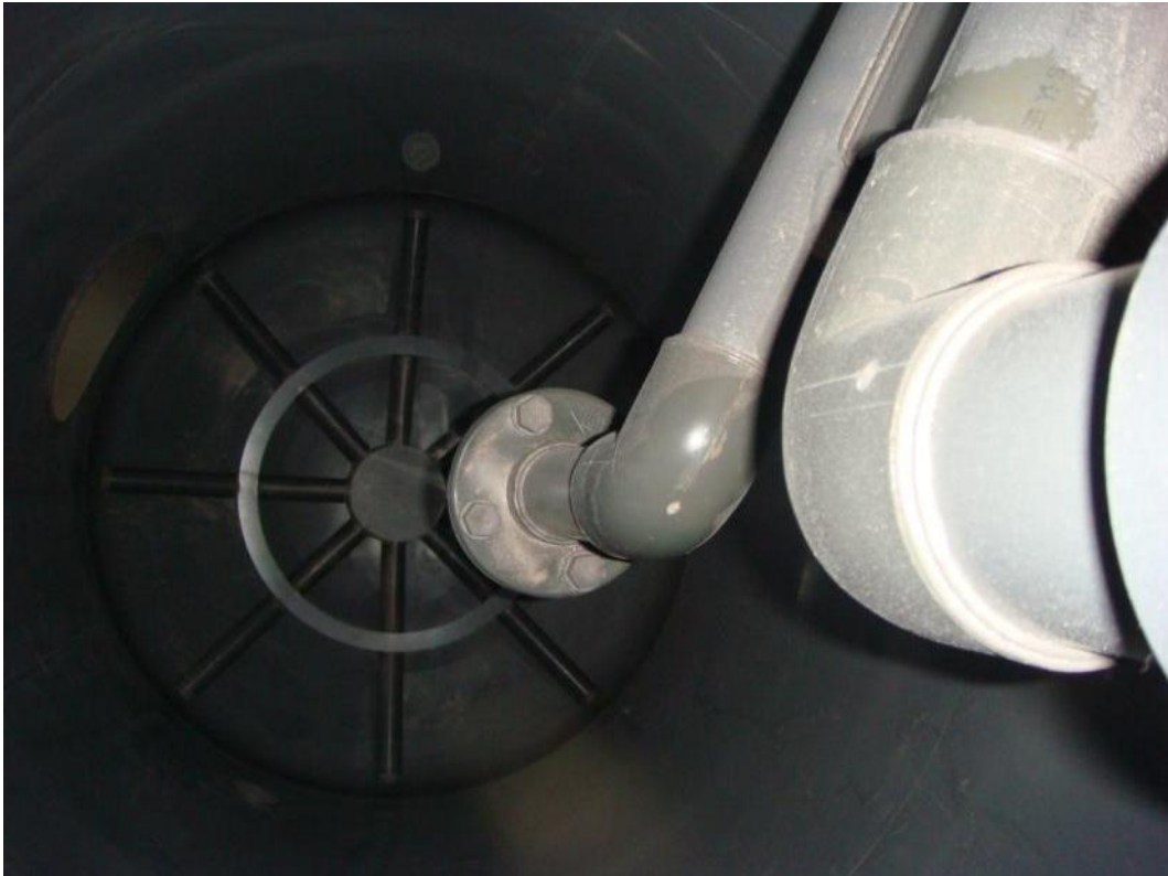
Tank Internal Piping
