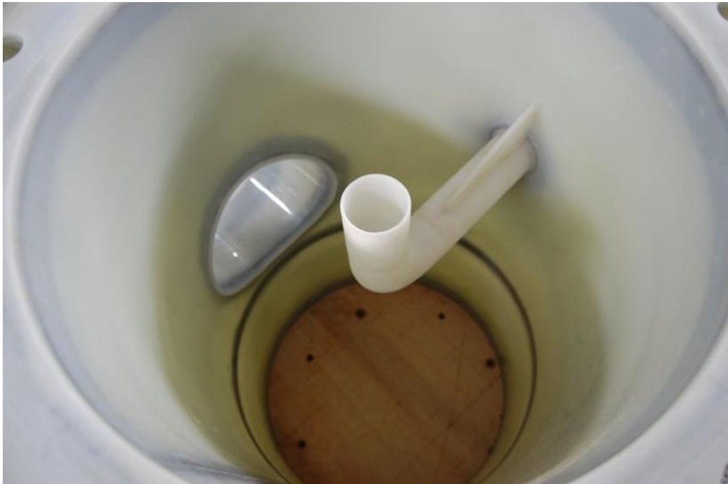
Tank Internal Pipe
